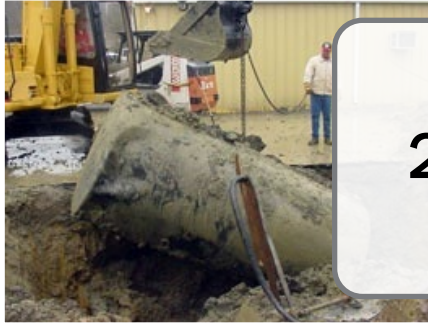
Underground Storage Tanks
